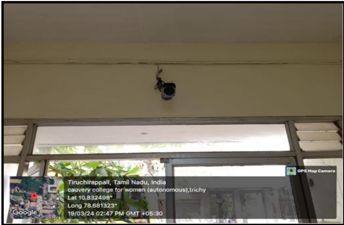
C – BLOCK GROUND FLOOR CORRIDOR CAMERA
