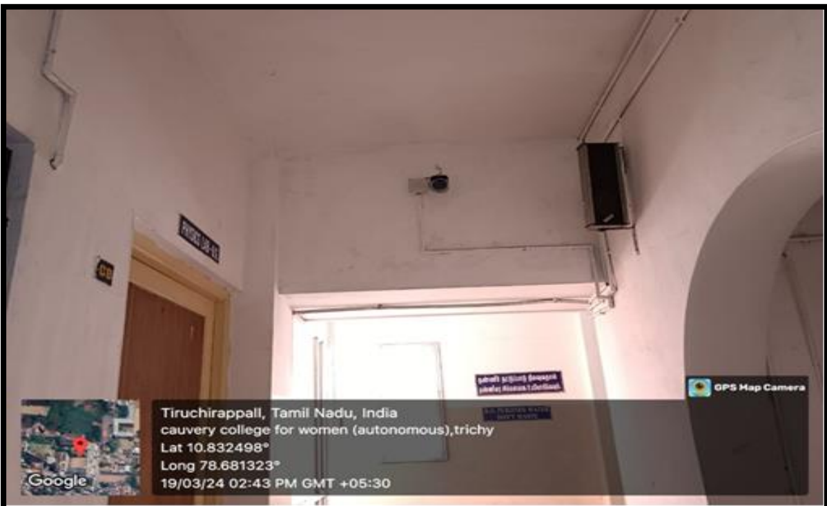
B – BLOCK FIRST FLOOR CORRIDOR CAMERA
