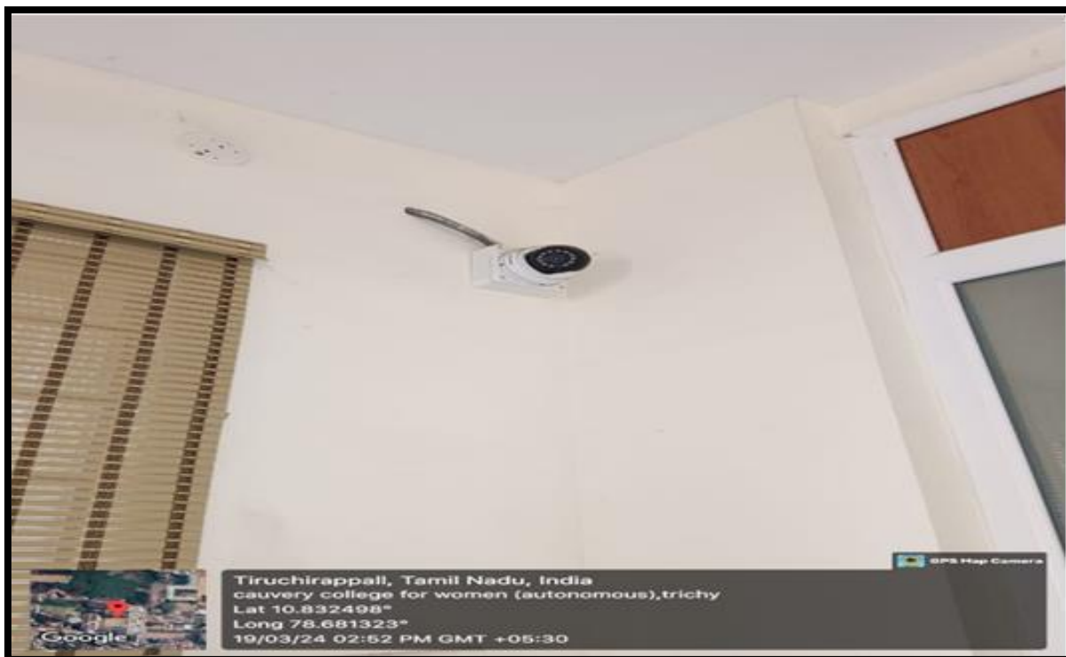
A – BLOCK GROUND FLOOR ENTRANCE - RECEPTION CAMERA
