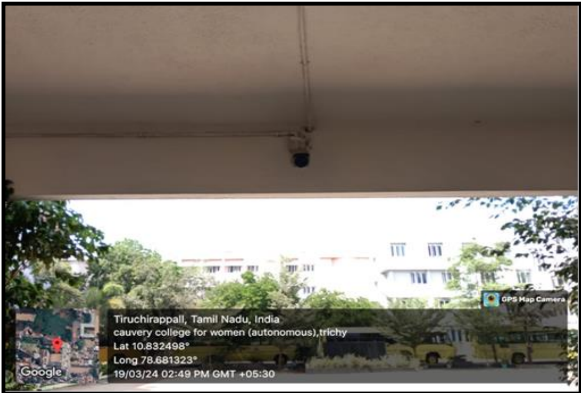
B – BLOCK GROUND FLOOR CORRIDOR CAMERA
